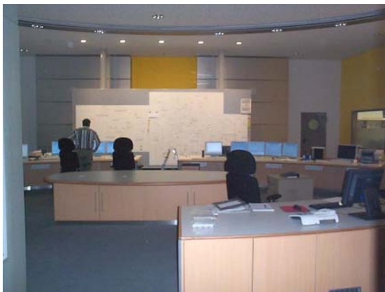
Leitwarte ENBW Ellwangen Central Controlroom ENBW Ellwangen (Germany)
